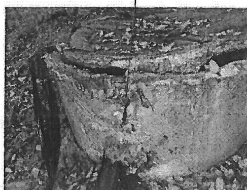
Damaged tank wall.
