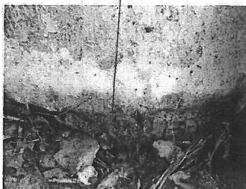
Sewage at damaged tank wall.
