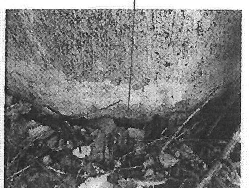
Damaged tank wall leak.
