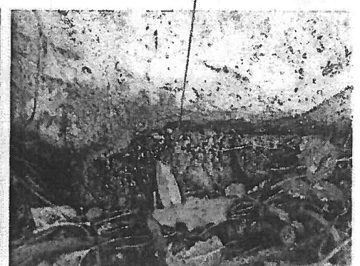
Sewage at damaged tank wall.
