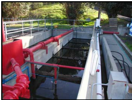
NBRID Treatment Plant
